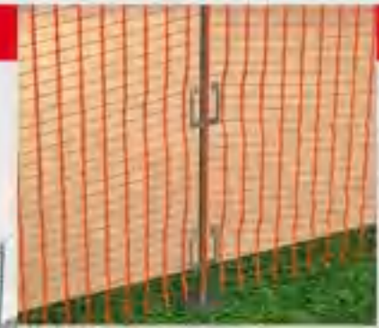
15. Mesh fencing system
